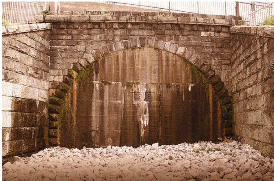
The sealed east entrance to the collapsed Church Hill Tunnel.
